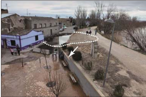
FIGURE 2. Image showing the location of the Alcalá sinkhole. The dashed line indicates the approximate limits of the area affected by higher subsidence. Arrow in the lower part of the image points to the northernmost fissure in the concrete wall. The photograph was taken on March 2, 2015, during the February-March Ebro River flood with a return period of 5-10 years. The water stage in the river is well above the ground surface in the village and water from the river was flowing under pressure through and beneath the dike, flooding the sinkhole
