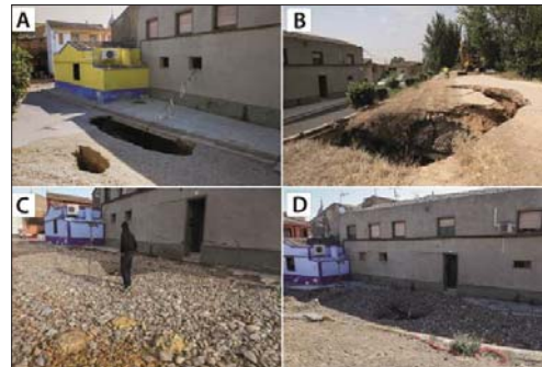
FIGURE 5. Photographs illustrating the evolution of the Alcalá sinkhole since 2007. A: Collapse sinkhole that reappeared in July 6, 2007, after filling a depression formed on June 20, 2007. Image taken on July 8, 2007. Note the lack of cracking in the adjacent buildings. B: Collapse sinkhole occurred in November 2013 on the eastern flank of the dike. C: Collapse-suffosion sinkhole formed soon after the compaction grouting program applied in the street with expansive polyurethane foam during November-December 2013. Note severe cracking in the adjacent buildings. Image taken on December 31, 2013. D: Collapse sinkhole on May 9, 2014
